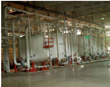
Chemical facility of the Zaporizhia NPP: central room of chemical water treatment
